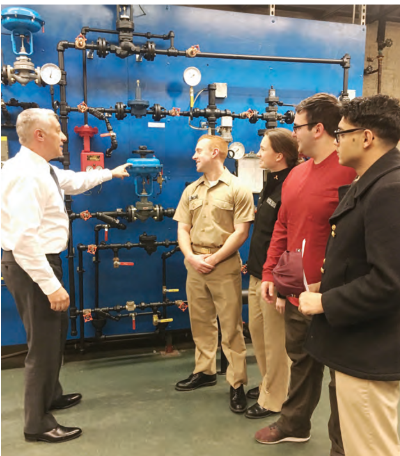
Joseph Lorino '87, an Adjunct Professor of engineering at SUNY Maritime College, teaches about steam pressure-reducing valves in the Analog Control Lab. Joe is also vice president, Facilities Management of the Valley Hospital based in Ridgewood, NJ.
